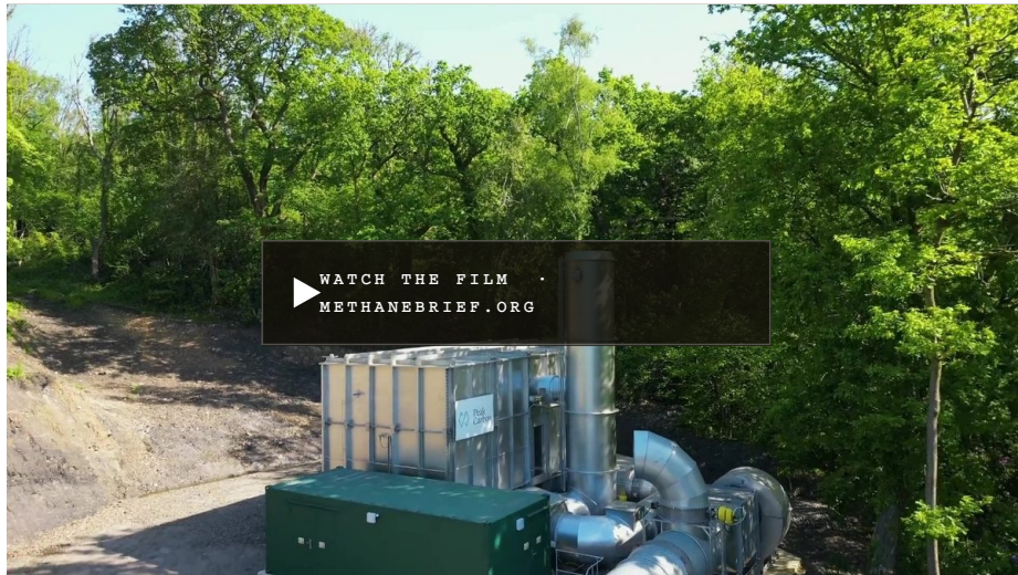
Aberpergwm Colliery, Glynneath, Wales: Peak Carbon's regenerative thermal oxidiser beside the ventilation shaft. Video: Peak Carbon.
