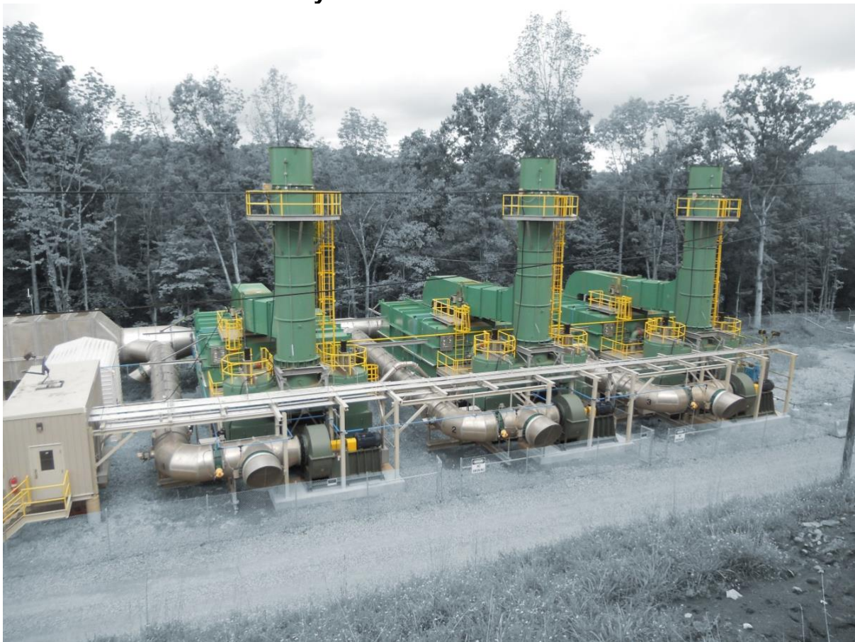
Ventilation Air Methane (VAM) mitigation, USA. Built 2012, operated more than 10 years. Considered for relocation. Picture courtesy of Durr CTS
