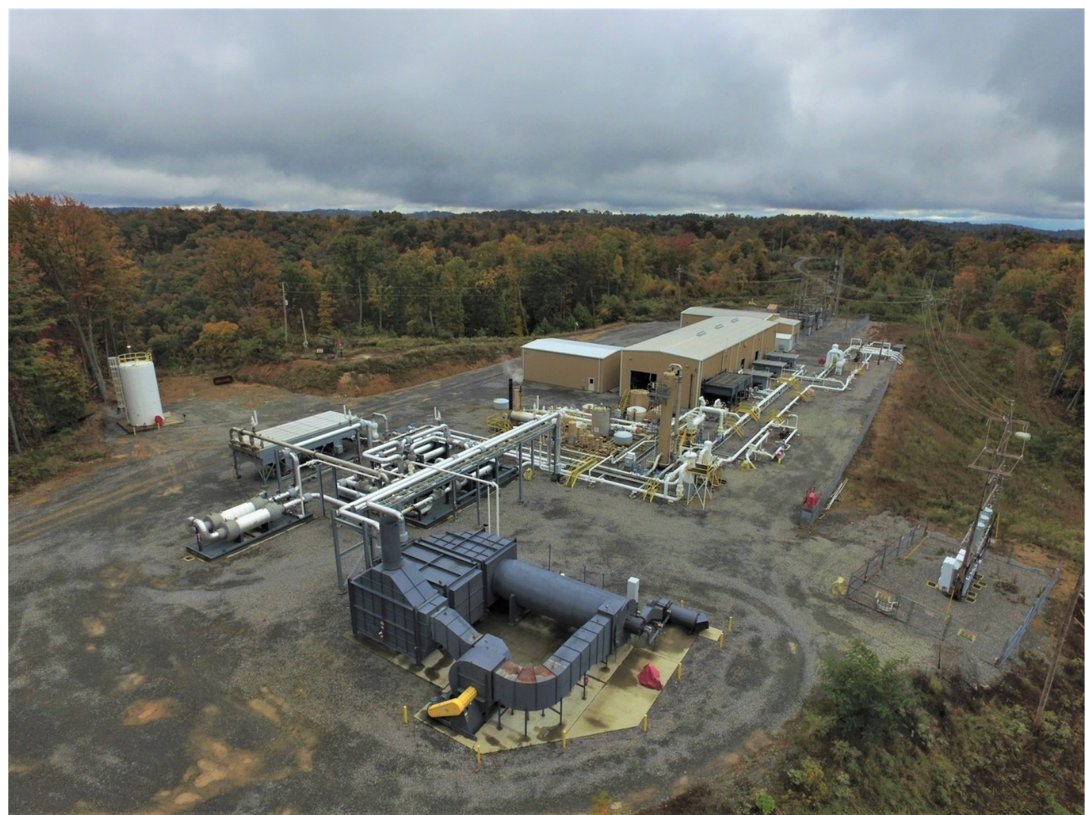
A CNX methane capture and processing facility in the Appalachian region. The dark unit in the foreground is a regenerative thermal oxidiser; processing and compression equipment runs along the site, feeding captured gas into the pipeline network. Courtesy of CNX Resources.
